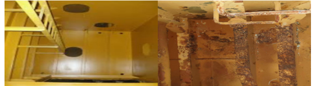
Fig. 1 Normal and corroded ballast tanks
