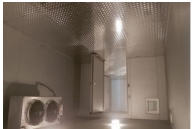
Fig. 1 Cold room for low temperature environment
